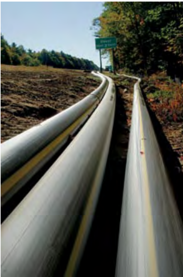
UNH’s innovative landfill gas project, EcoLine, includes a pipeline that runs 12.7 miles from Waste Management’s Turnkey Recycling and Environmental Enterprise facility in Rochester to the campus in Durham.
